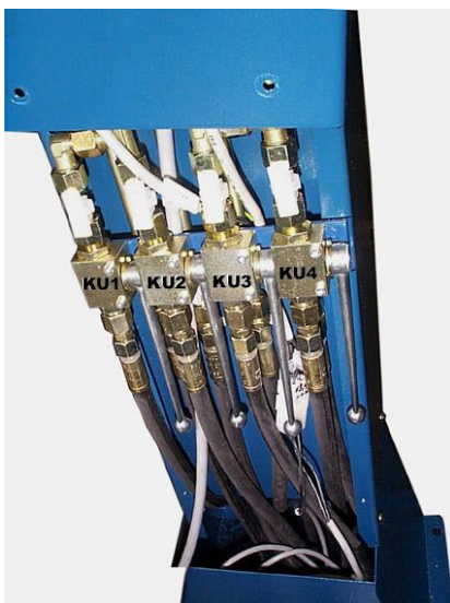
pic. 2: ball valves for the equalization of the lift.
